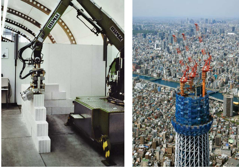
FIGURE 1.4: On-site construction robots and automated construction site. (a) Thomas Bock, ESPRIT 3 6450 ROCCO (RObotic Computer integrated CONstruction) masonry robot, Karlsruhe University, Germany, 1992–6: Development of a mobile heavy-duty robot for the construction sector, here applied to robotic on-site assembly Bock and Langenberg, 2014. (b) Nikken Sekkei, Tokyo Sky Tree, partly automated construction site, Tokyo, 2010: The 32-storey, 634-metre (2,080-foot) tall Tokyo Sky Tree radio and television tower in the city centre was built and is operated by Obayashi Corp.. (Bock and Langenberg, 2014)
